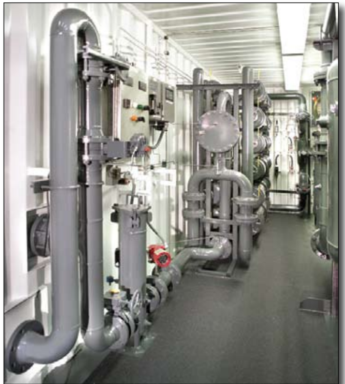
Interior View of Containerized System
